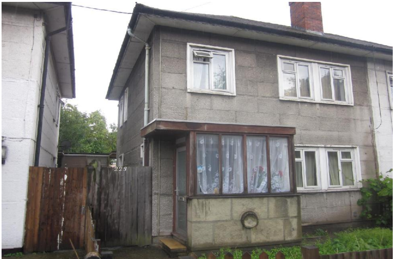
Photograph C19 – Example of no finishes to cladding and porch extension
