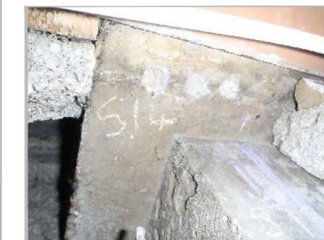
PA11d: VIEW LOOKING UP AT PRIMARY ROOF BEAM BEARING ONTO COLUMN HEAD AT EXPOSURE EXP A3
