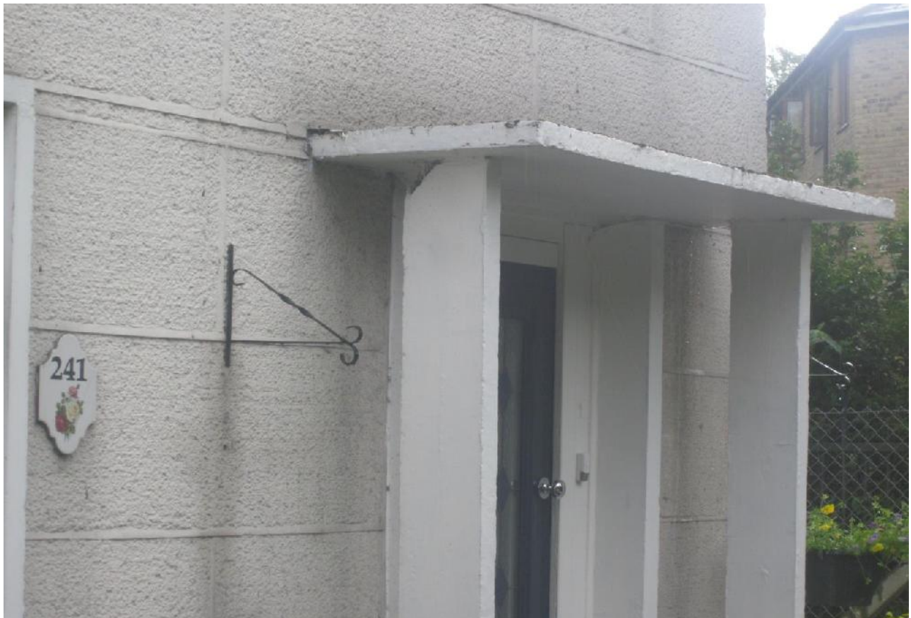
Photograph C23 – Canopy support spalling
