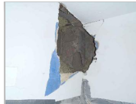
PD6a: VIEW OF 1ST FLOOR COLUMN. NOTE PHOTO TAKEN POST REINSTATEMENT OF B/O D1
