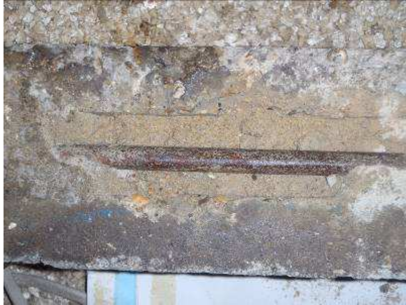
Plate R8: View of Breakout D2 to roof secondary beam continuity bar over central column at No. 20 Hatfield Close.
