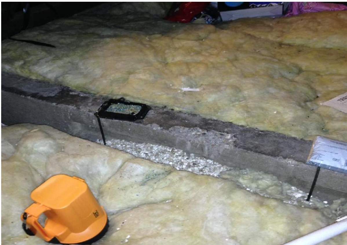
Photograph C6 – Damage to secondary beam
