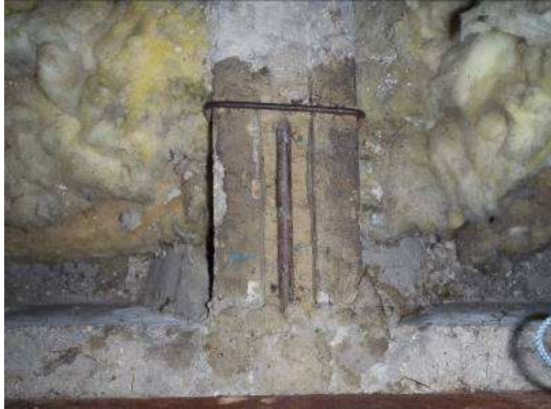
Plate R2: View of Breakout C1 to continuity bar at roof secondary beam to roof primary beam connection over central column at No. 1 Rutter Gardens.
