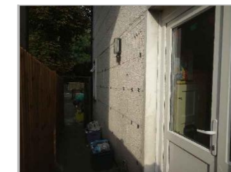
PB.14a: VIEW OF WALL TIE SURVEY AREA B1 ON WESTERN SIDE OF PROPERTY AT GROUND FLOOR LEVEL
