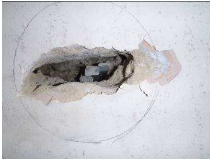
Plate R9: View of tie fishtail end embedded within internal blockwork skin at Breakout D6 to No. 20 Hatfield Close.
