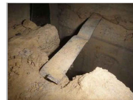
PB10b: VIEW OF B/O B4 TO WALL TIE EMBEDMENT WITHIN INTERNAL BLOCKWORK SKIN
