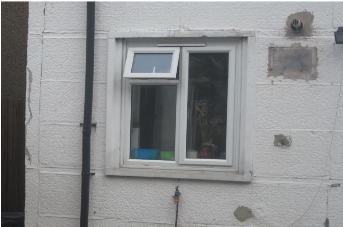
Photograph C9a – Spalled corner cladding panel and covered venting cladding panel to rear of 193 Morden Road
