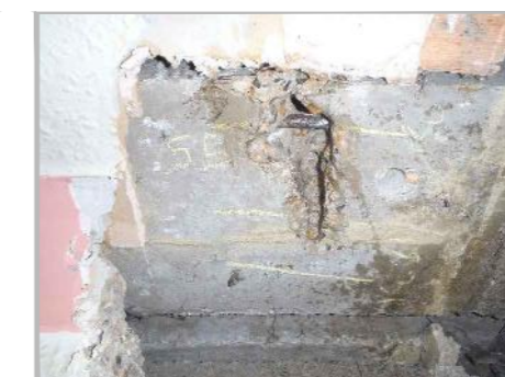
PA6b: VIEW LOOKING UP AT B/O A3 TO SOFFIT OF PRIMARY ROOF BEAM
