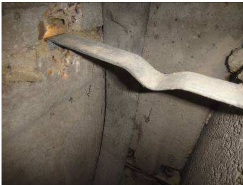
Fig. R5: View of Breakout B3 to tie embedment within external cladding panel at No. 193 Morden Road.
