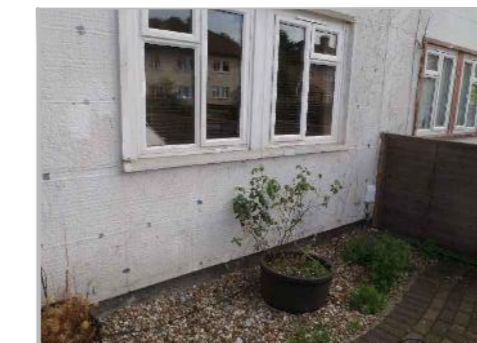
PD9a: PART VIEW OF SOUTHERN SIDE OF WALL TIE SURVEY AREA D1
