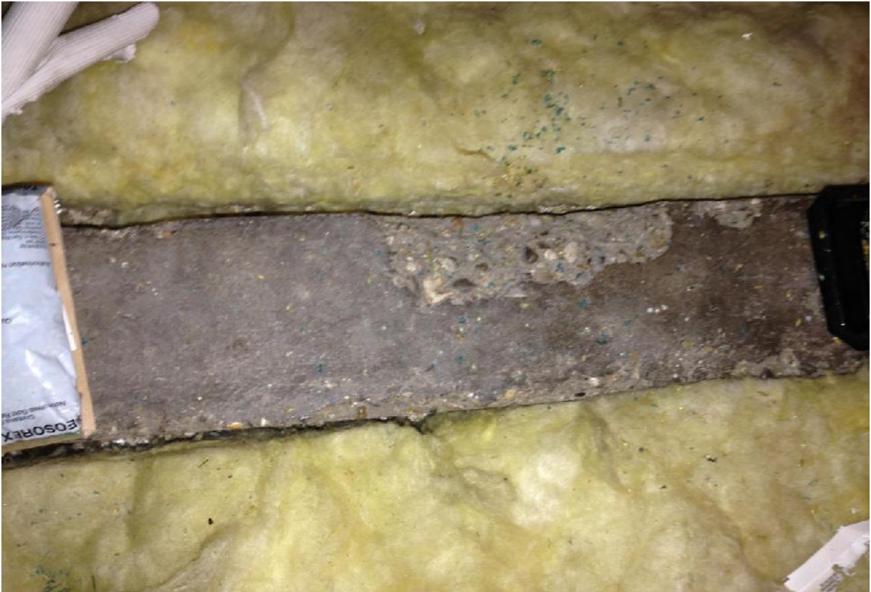
Photograph C3 – Damage to secondary beam
