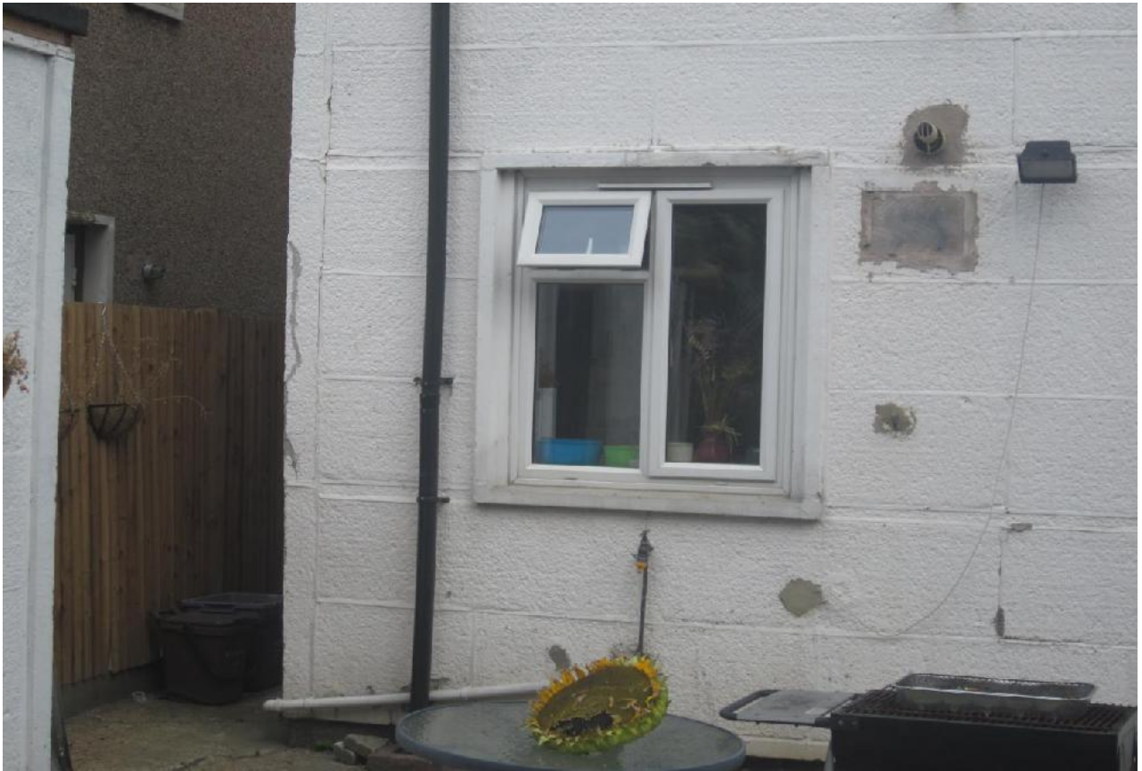
Photograph C9 – Spalled corner cladding panel and covered venting cladding panel to rear of 193 Morden Road
