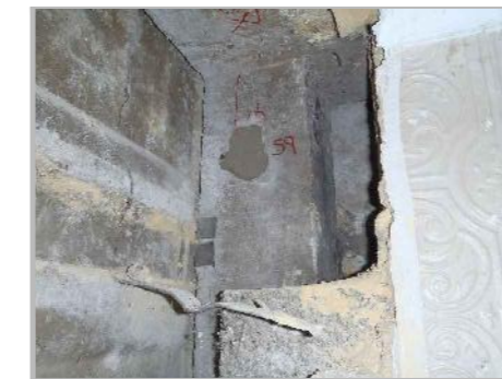
PA9b: CLOSER VIEW OF COLUMN HEAD AND SOFFIT OF ROOF PRIMARY BEAM AT EXPOSURE EXP A1
