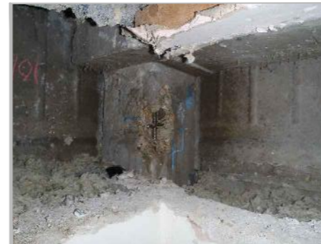
PD5a: VIEW OF B/O D1 TO GROUND FLOOR COLUMN. NOTE INSULATION WITHIN CAVITIES.
