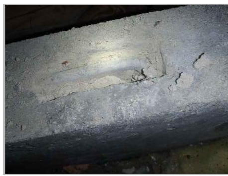
PA4a: VIEW OF B/O A5 TO CONTINUITY BAR WITHIN TOP OF SECONDARY BEAM
