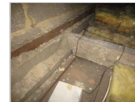
PB3b: SECONDARY BEAM BEARING ONTO EASTERN PRIMARY BEAM. NOTE CHANGE IN BEAM SECTION. PREFORMED SLOT WITH NO CONTINUITY BAR AND MORTAR HAUNCH AT BEAM BEARING.
