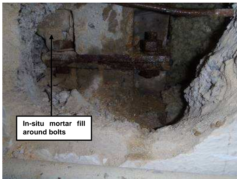
Plate R4: View of Ground Floor to 1 st Floor column connection at No. 1 Rutter Gardens. Note in-situ mortar fill around bolts partially removed for inspection.
