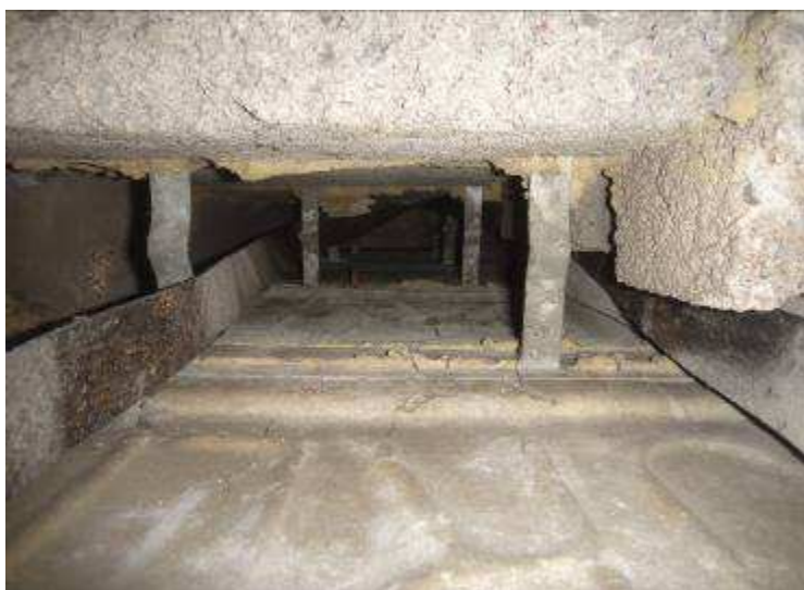
Plate R6: View looking up towards cavity wall ties above Breakout B3 at No. 193 Morden Road.
