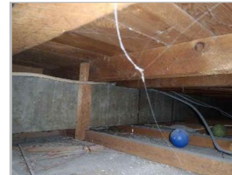
PD5b: VIEW LOOKING SOUTH FROM B/O D1 WITHIN 1ST FLOOR CEILING VOID
