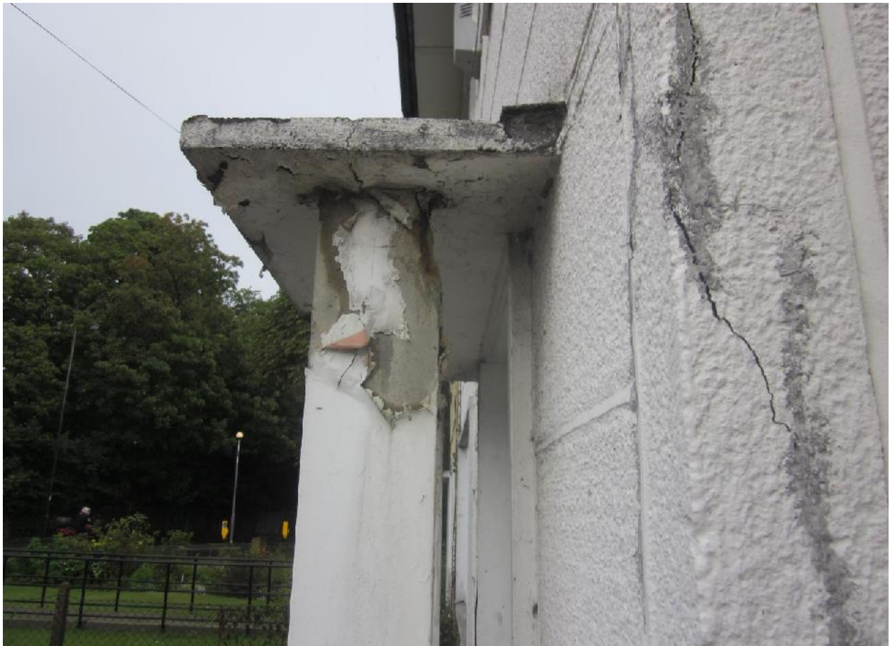
Photograph C16 – Example of corner cladding and canopy support spalling
