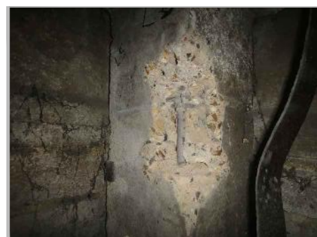
PB11a: VIEW OF B/O B5 TO GROUND FLOOR COLUMN AT LOW LEVEL
