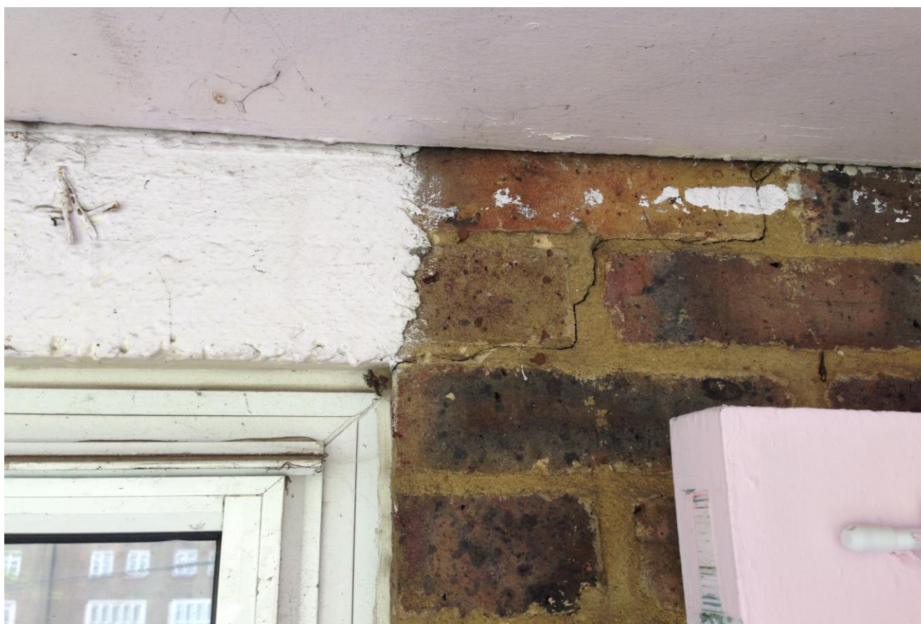
Photograph C4 – 1-3mm Crack in Mortar Above Window on 14 Ravensbury Grove External Terrace
