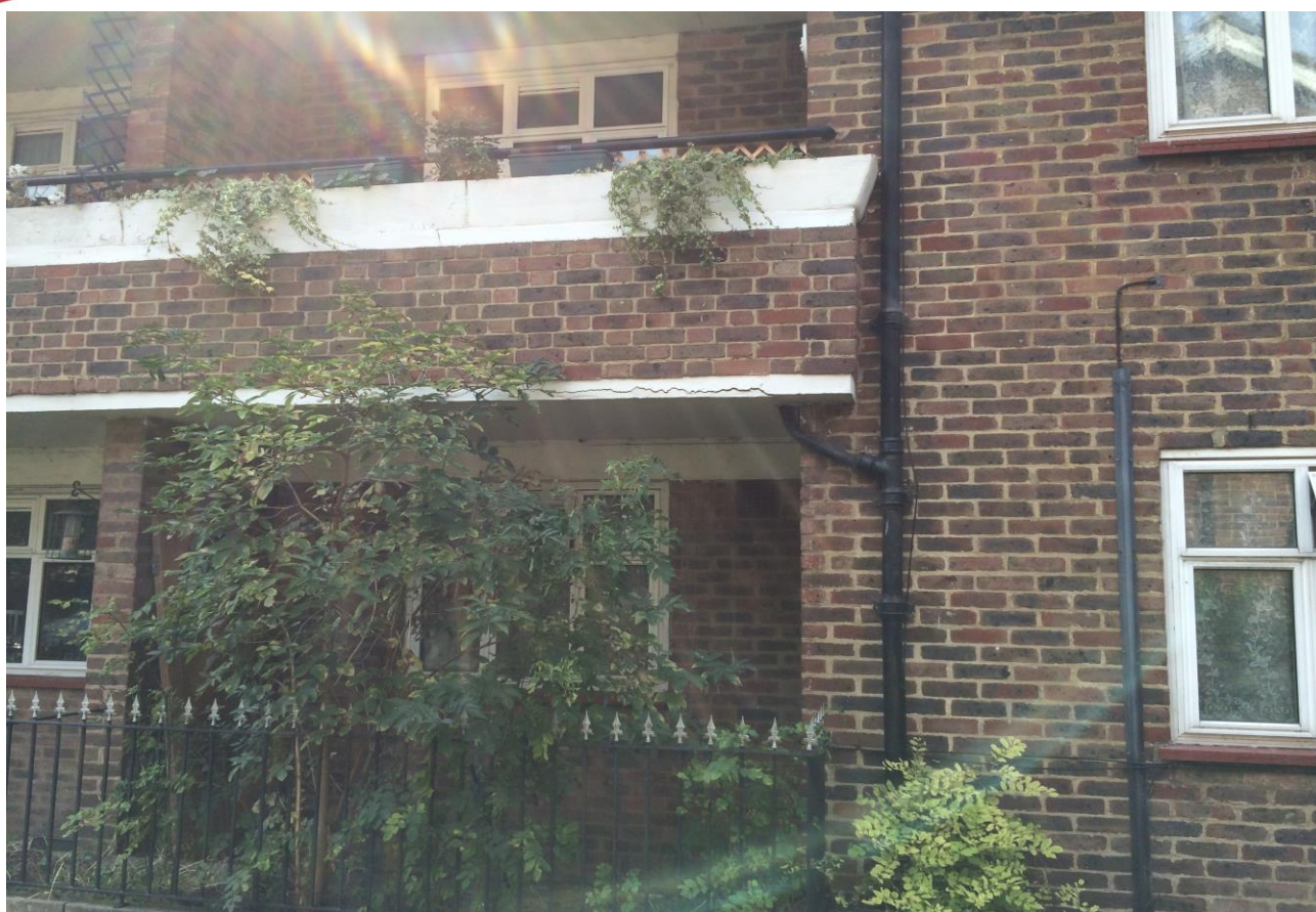
Photograph C3 – 1-6mm Horizontal Crack in Terrace Soffit
