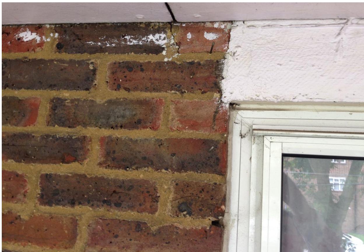
Photograph C5 – 1-3mm Crack Above Window on 14 Ravensbury Grove 's External Terrace
