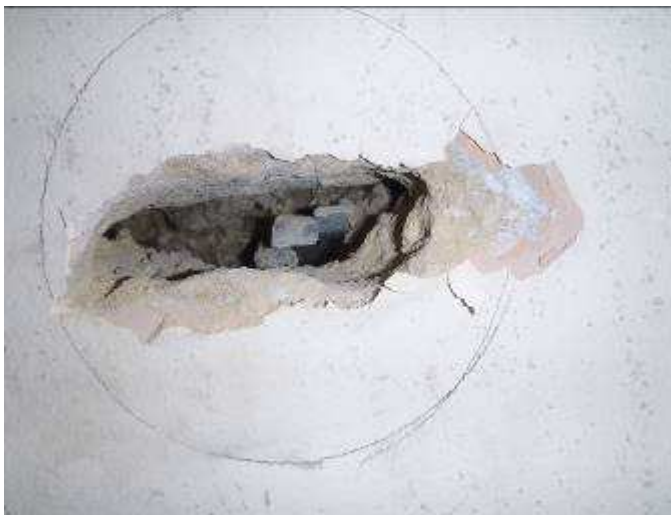
Plate R9: View of tie fishtail end embedded within internal blockwork skin at Breakout D6 to No. 20 Hatfield Close.
