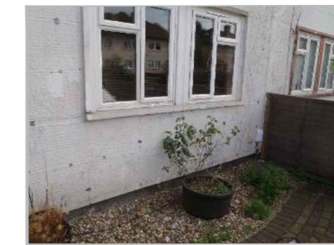
PD9a: PART VIEW OF SOUTHERN SIDE OF WALL TIE SURVEY AREA D1
