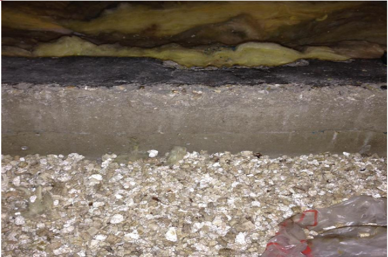
Photograph C7 - Damage to secondary beam
