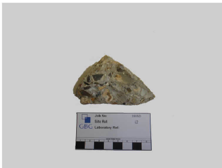
Plate R11: View of concrete lump sample L2D from a 1 st Floor secondary beam at No. 20 Hatfield Close.
