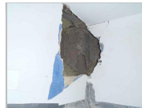
PD6a: VIEW OF 1ST FLOOR COLUMN. NOTE PHOTO TAKEN POST REINSTATEMENT OF B/O D1
