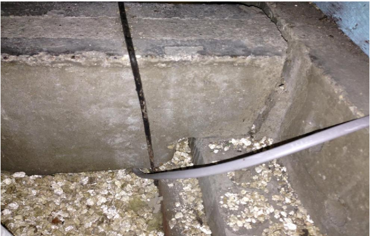
Photograph C2 – Discontinuity of mortar/concrete between primary beam and secondary beam connection
