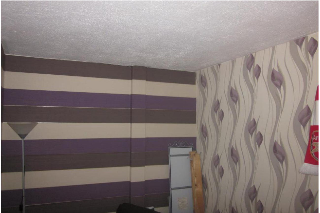
Photograph C10 – Evidence of internal column projection on party wall line into room
