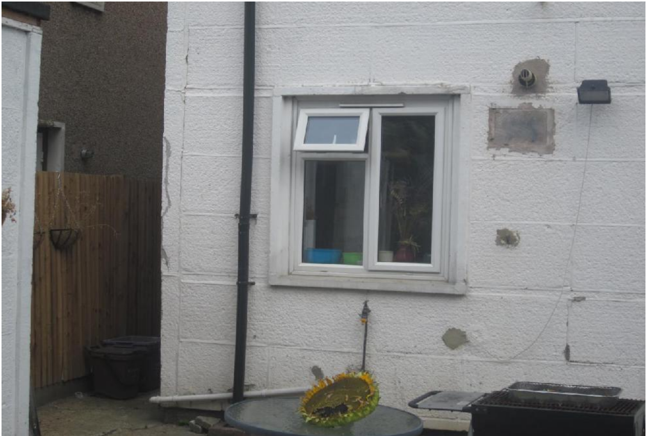
Photograph C9 – Spalled corner cladding panel and covered venting cladding panel to rear of 193 Morden Road
