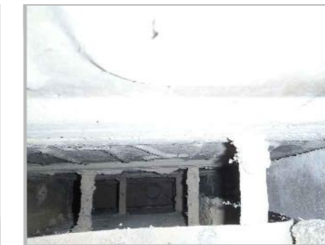
PA9c: VIEW LOOKING DOWN CAVITY ADJACENT TO 1ST FLOOR COLUMN AT EXPOSURE EXP A1
