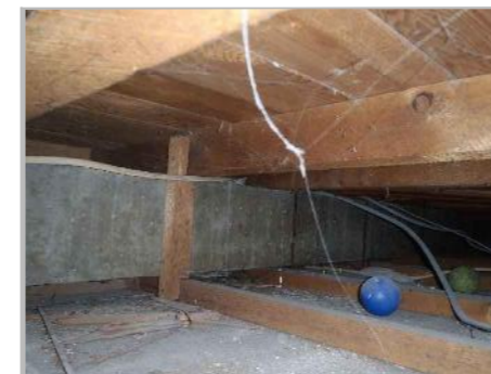
PD5b: VIEW LOOKING SOUTH FROM B/O D1 WITHIN 1ST FLOOR CEILING VOID
