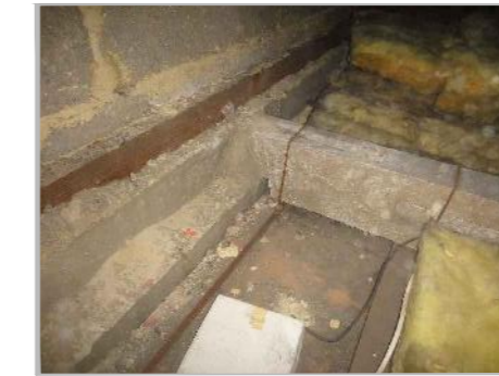
PB3b: SECONDARY BEAM BEARING ONTO EASTERN PRIMARY BEAM. NOTE CHANGE IN BEAM SECTION. PREFORMED SLOT WITH NO CONTINUITY BAR AND MORTAR HAUNCH AT BEAM BEARING.
