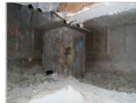
PD5a: VIEW OF B/O D1 TO GROUND FLOOR COLUMN. NOTE INSULATION WITHIN CAVITIES.
