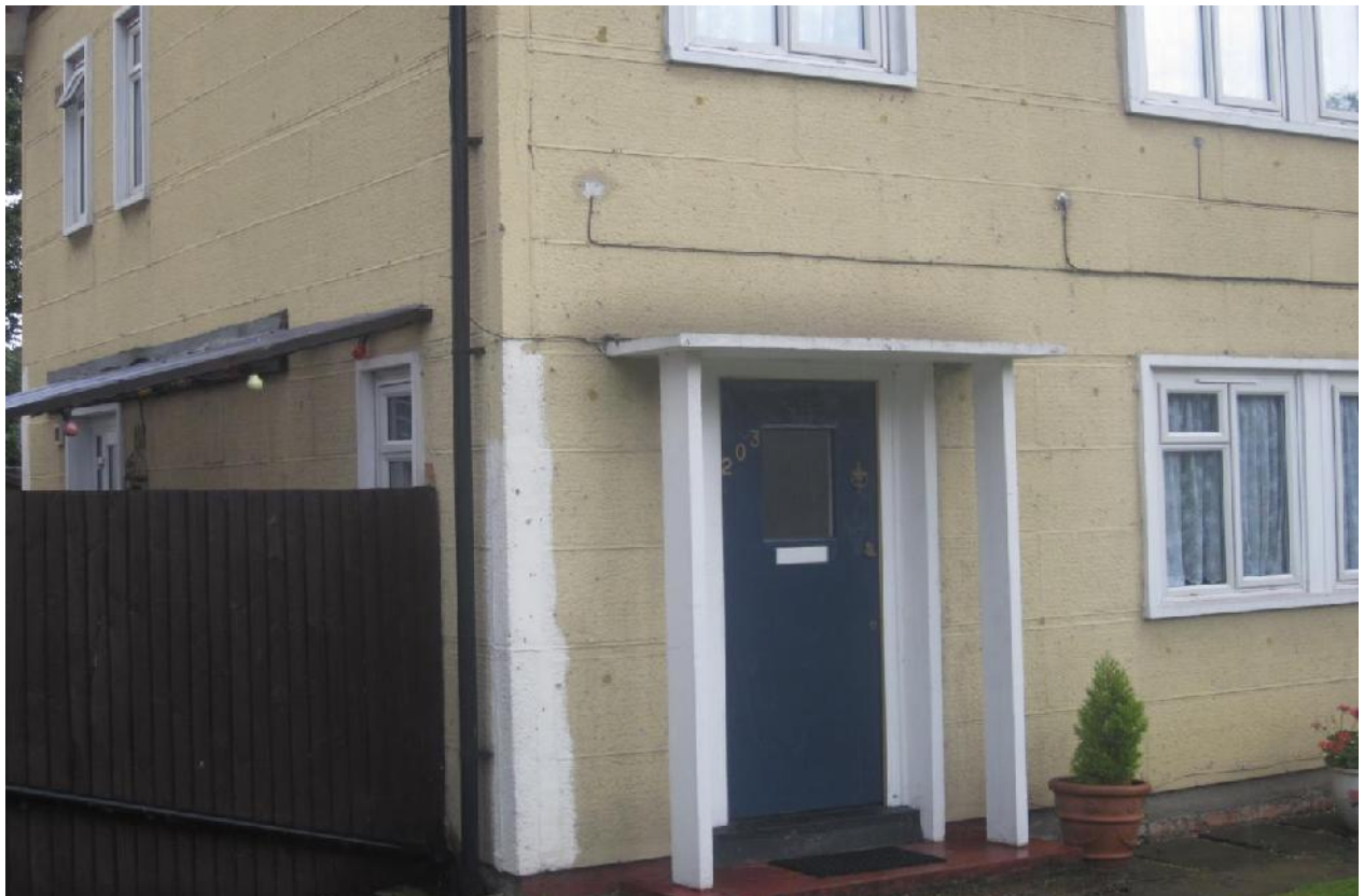
Photograph C15 – Evidence of corner cladding repair
