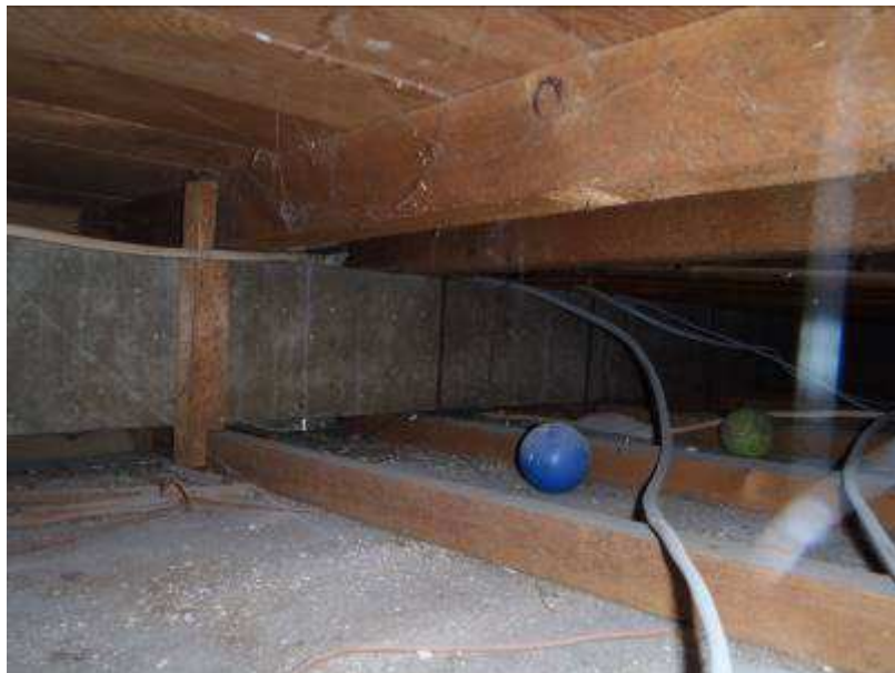
Plate R3: View of typical 1 st Floor structure at No. 20 Hatfield Close
