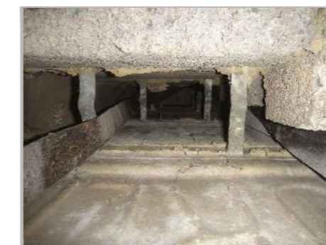
PB10c: VIEW LOOKING UP WITHIN CAVITY WALL ON EASTERN SIDE OF COLUMN AT B/O B4
