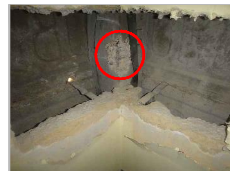
PB12a: VIEW OF B/O B6 TO GROUND FLOOR COLUMN AT HIGH LEVEL. NOTE ALSO EXPOSED WALL TIES
