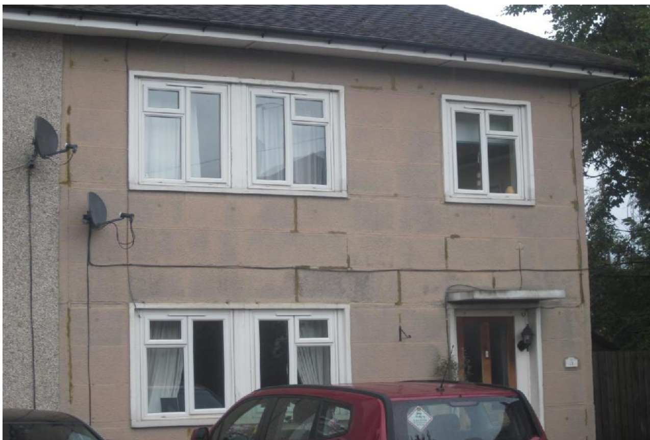
Photograph C27 - Significant mortar repair
