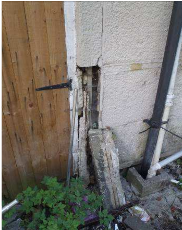
Plate R10: View of spalled corner panel at ground floor level to No. 1 Rutter Gardens
