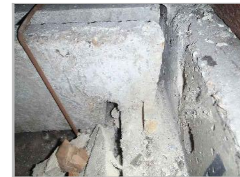
PA3a: VIEW OF SECONDARY BEAM BEARING ONTO PRIMARY BEAM AT SECTION AA-AA POST REMOVAL OF MORTAR HAUNCH
