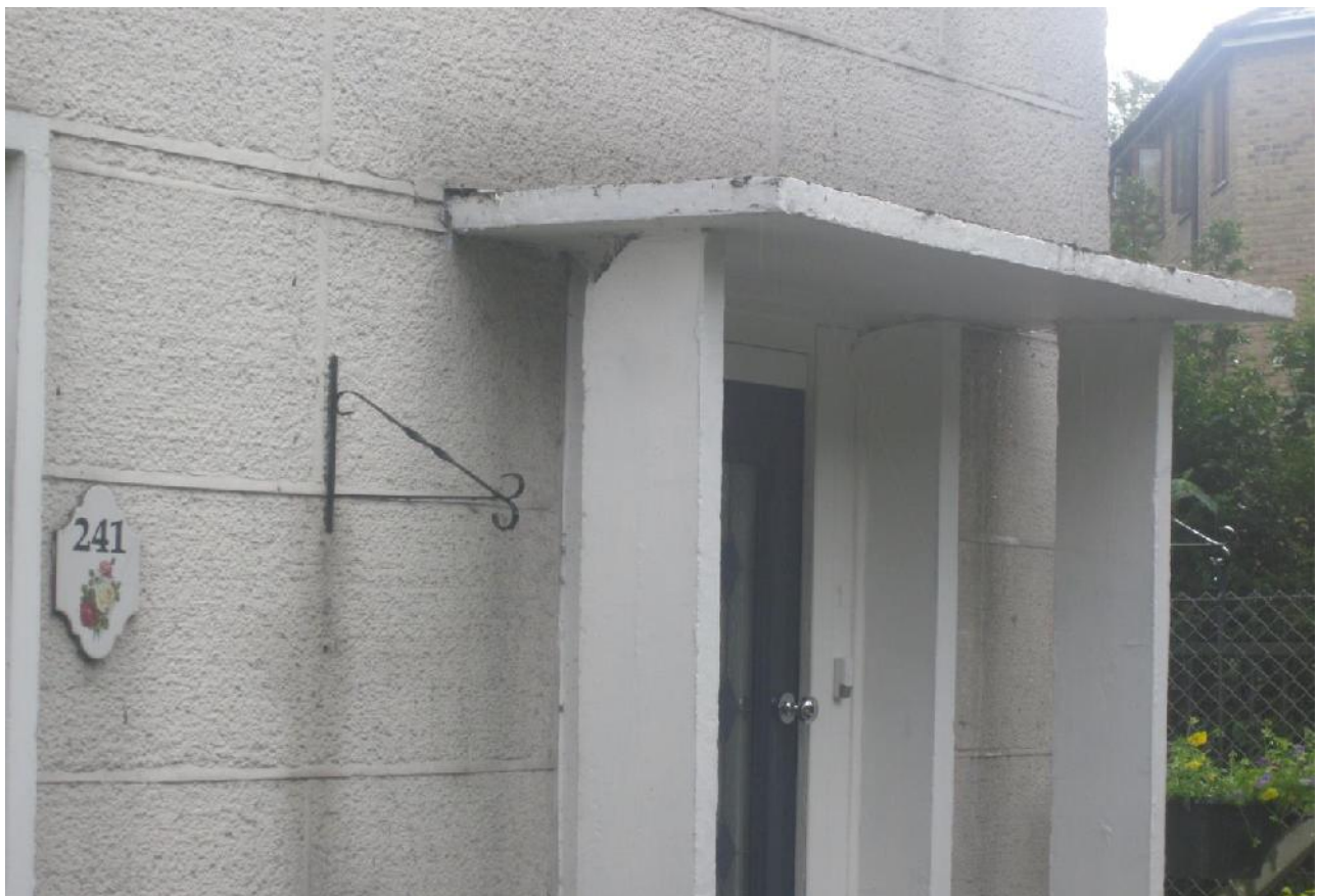
Photograph C23 – Canopy support spalling
