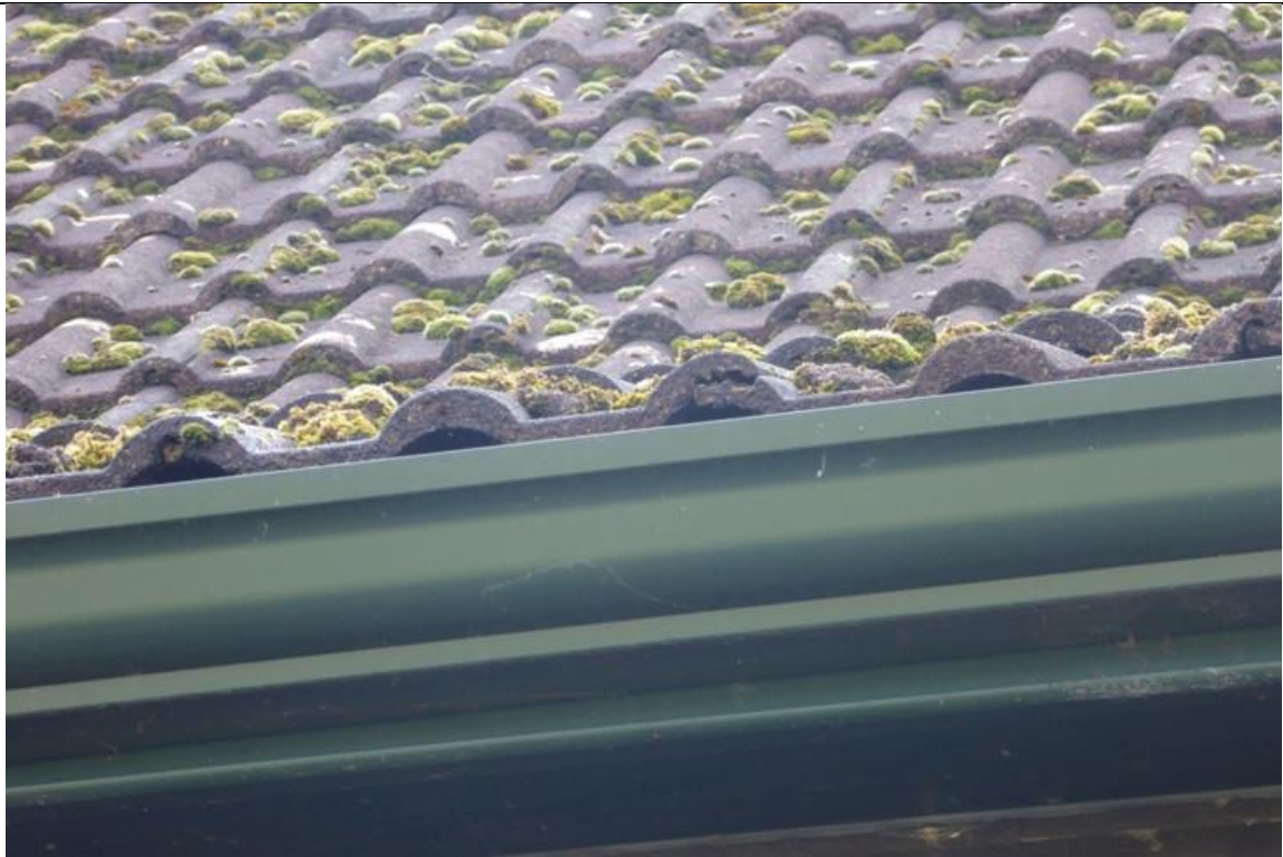
Photo 3: Bowls Pavilion (Building B) – note gaps under tiles at the roof edge
