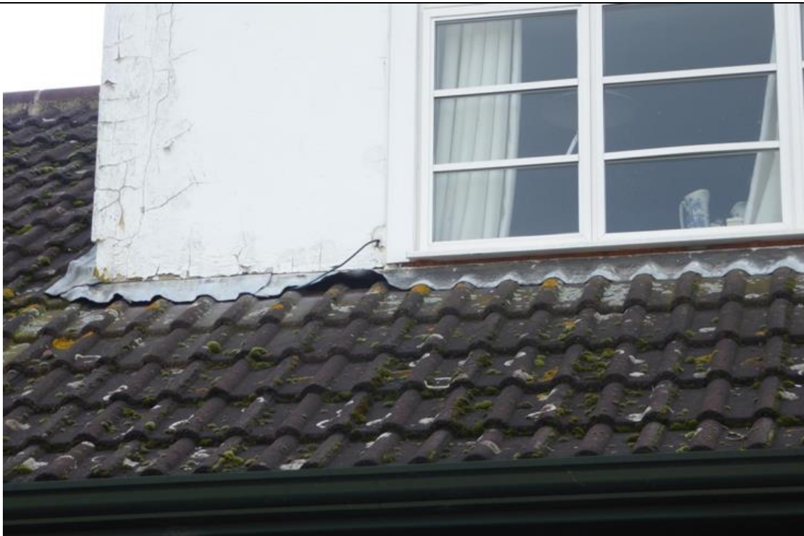
Photo 2: Bowls Pavilion (Building B) – note raised flashing
