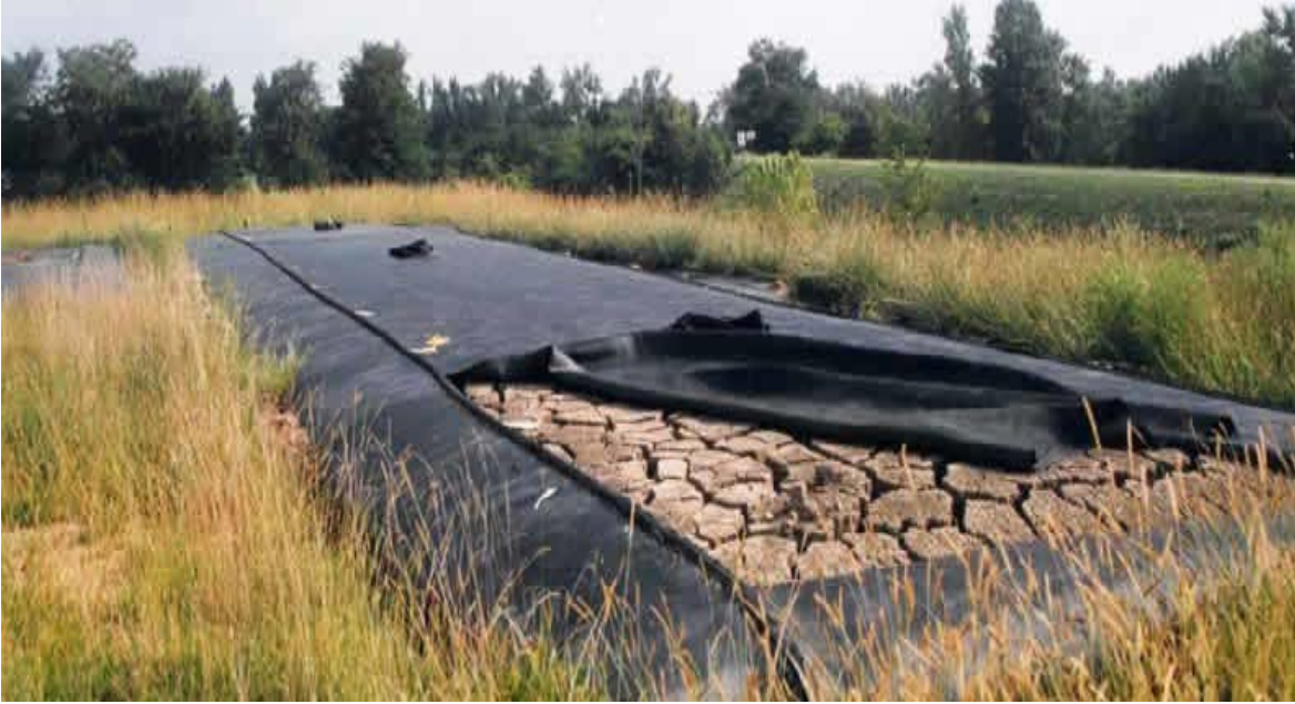
Dried silts being cut from the silt bags to be used in landscaping.
