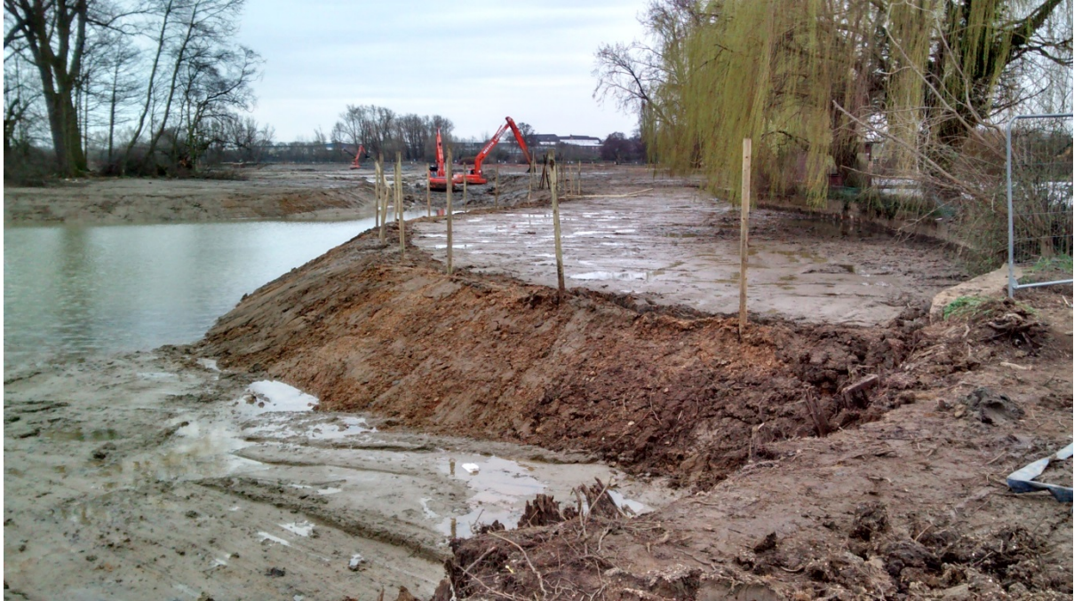
Excavation of the lake bed subsoils in order to create bunds, behind which dredged silts are stored.
