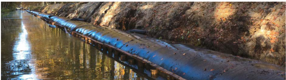
Dredged silts stored in the silt bags at a greater depth and density than when loose in the water body.
