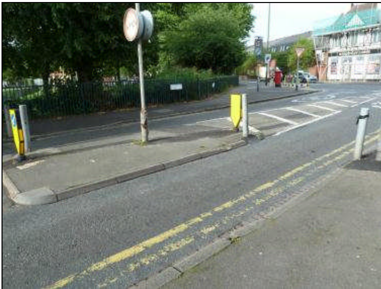
Crossing CR638X Quicks Road west of Haydon's Road – dropped kerbs on footways but not island (also no tactile paving)
