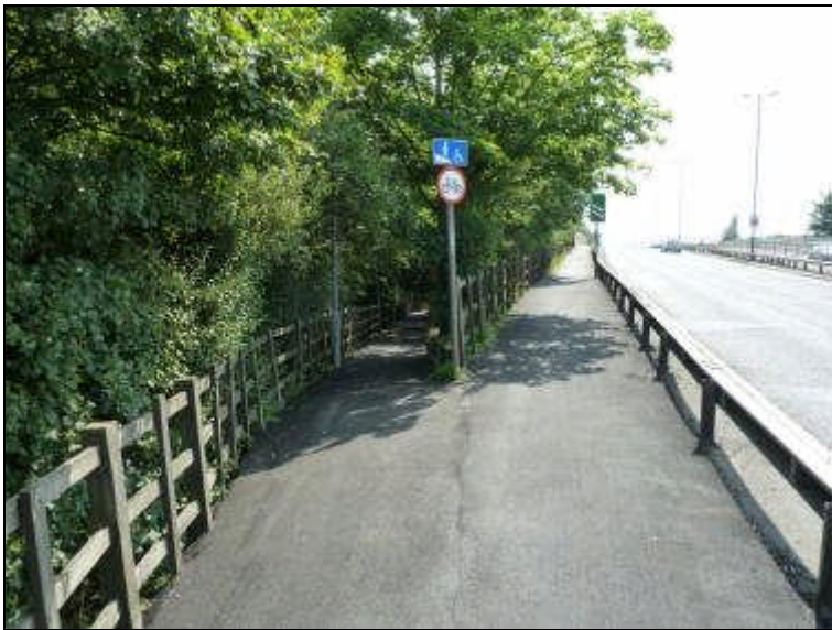
Ramp from A3 footway to eastern end of Aboyne Drive subway (CR499)
