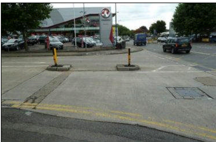
Crossing CR621 Waterside Way junction with Plough Lane (1.2m refuge, intended for shared use by cyclists and pedestrians!)
