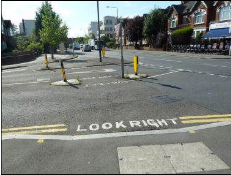
Crossing CR780: Cannon Hill Lane at junction with Kingston Road (NB no tactile paving)
