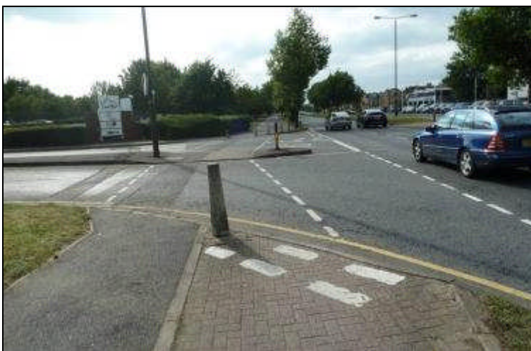
CR788 David Lloyd Centre access road junction with Bushey Road – cycle track crossing not aligned with island (and bollard makes situation worse)
