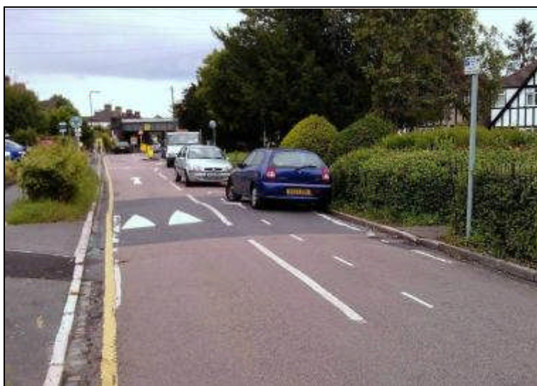
Crossing CR445 Toynbee Road – paths on both side but only one dropped kerb
