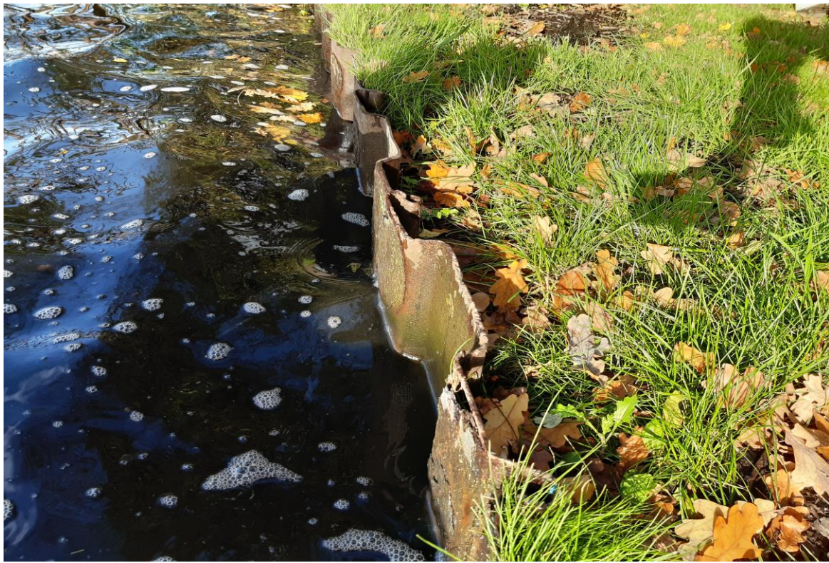
Plate 13 Area of sheet pile where timber fendering and metallic capping is not present
