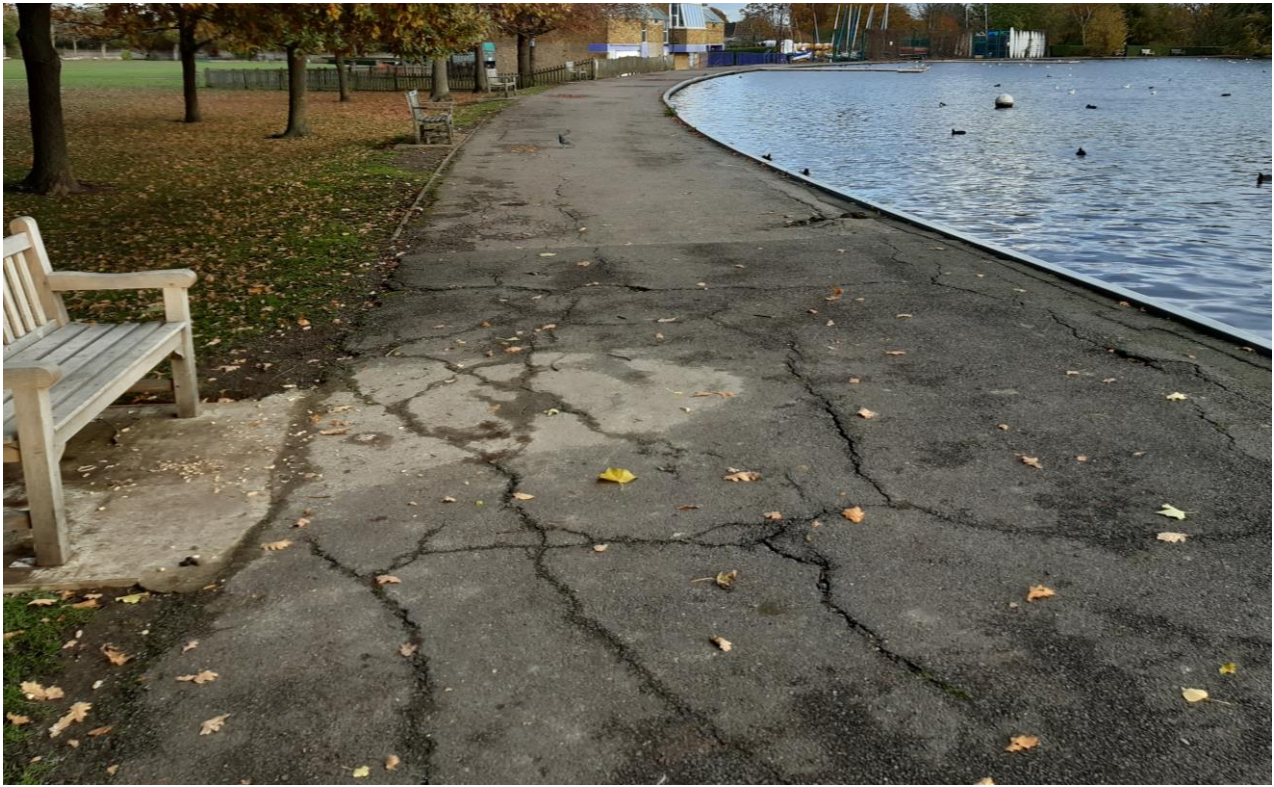
Plate 9 View east showing cracks in asphalt in the north area of the site
