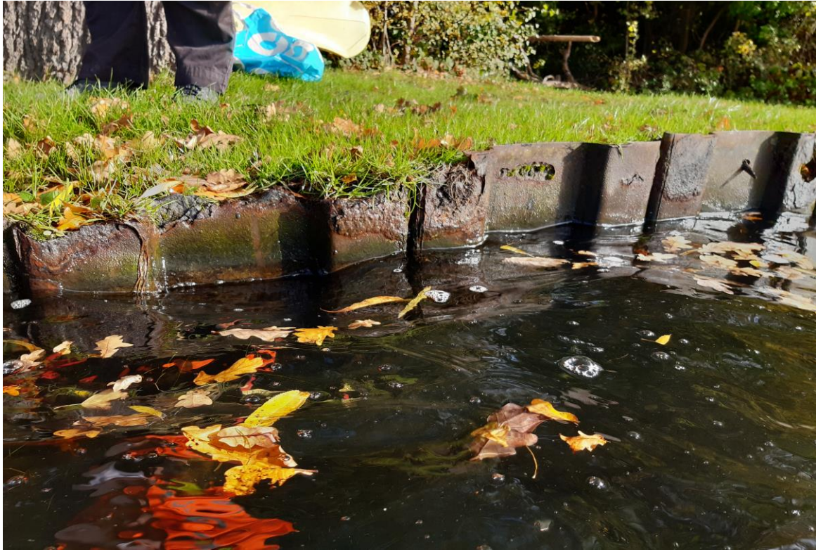
Plate 25 Evidence of corrosion on sheet pile at fishing bank
