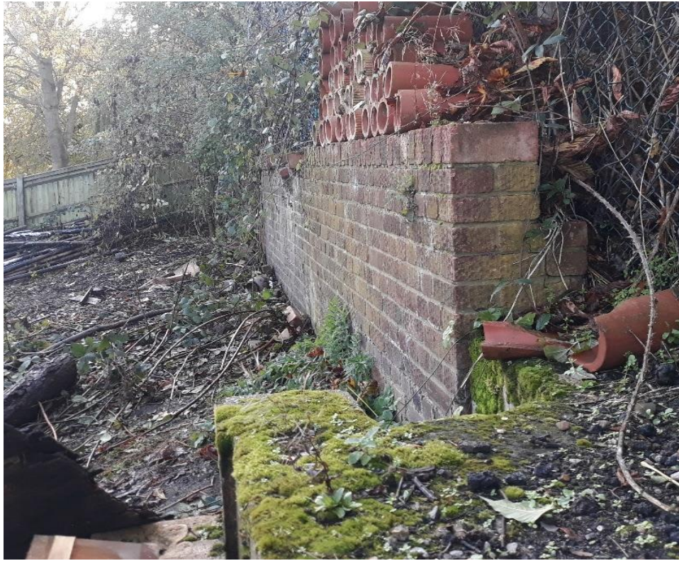
Plate 15 View along the retaining wall from the top of the adjacent blockwork wall
