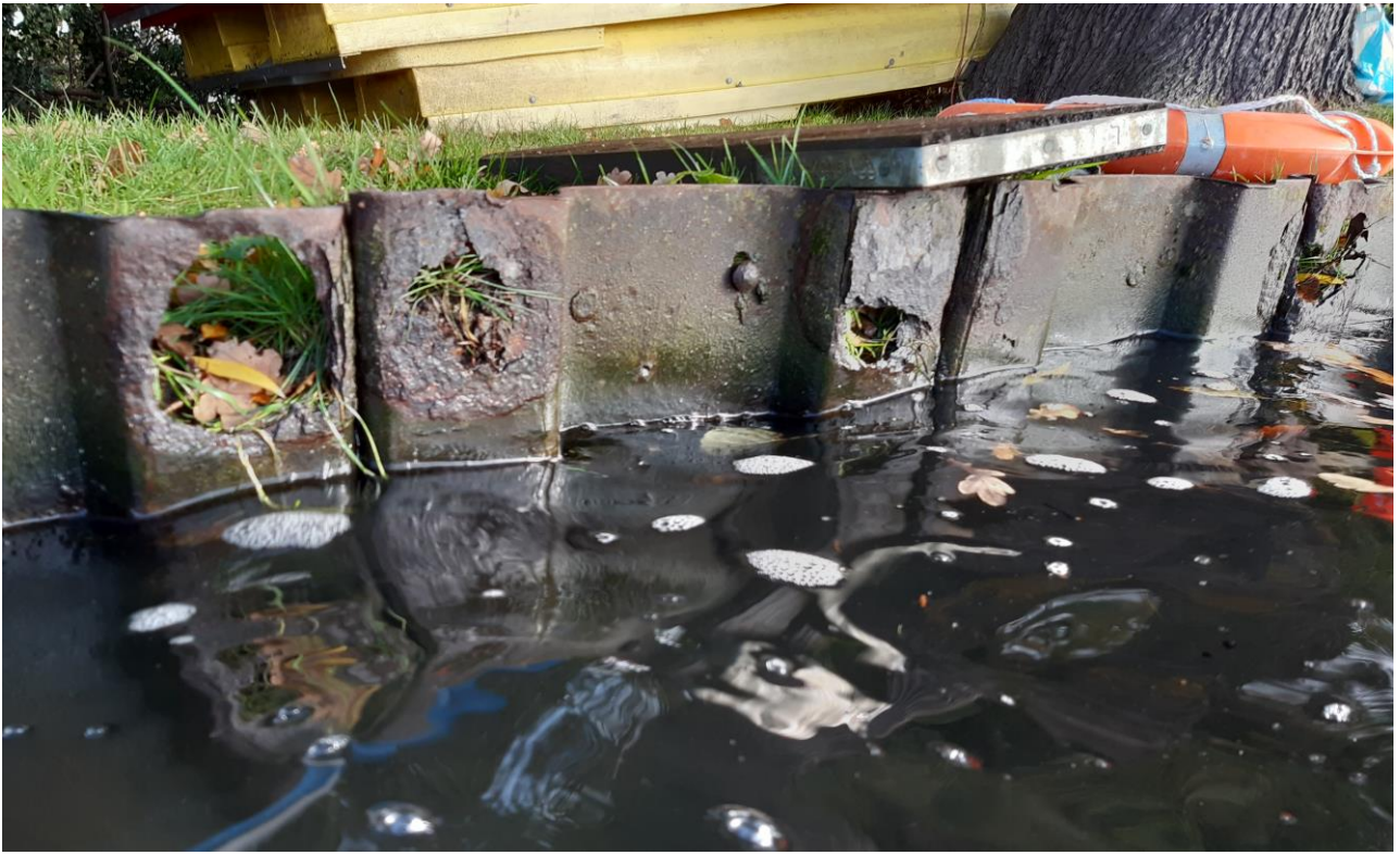
Plate 23 Organic growth and minor defects on sheet pile on fishing bank
