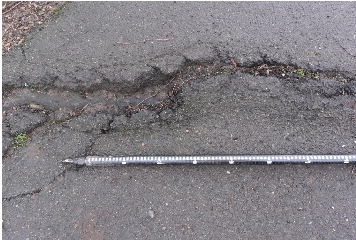
Plate 11 Damage to the asphalt due to root breaching in the central east area of the site
