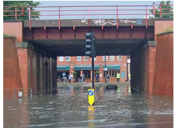
Flooding of Raynes Park Railway Bridge, July 2007
