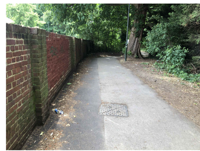
EXISTING SHARED USE PATH SHOWING WALL TO BE REMOVED AND EXISTING LAMP POST
