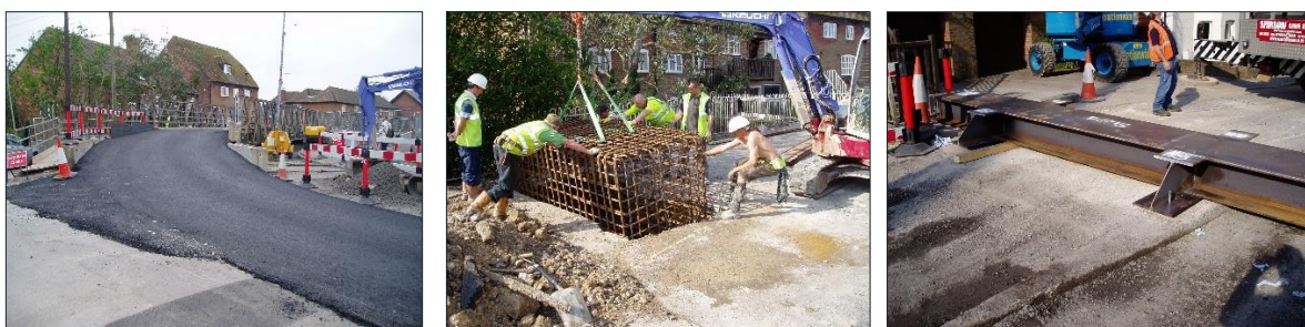
Figure 46 - (L) Temporary ramp construction (C) Temporary bridge, in-carriageway construction (R) Trimmer beam used to achieve elevation above deck level
