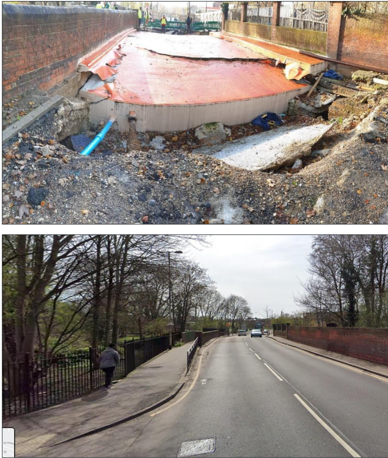
Figure 5 - View across structure towards south [Top - current view following collapse, Bttm – view prior to strengthening works]
