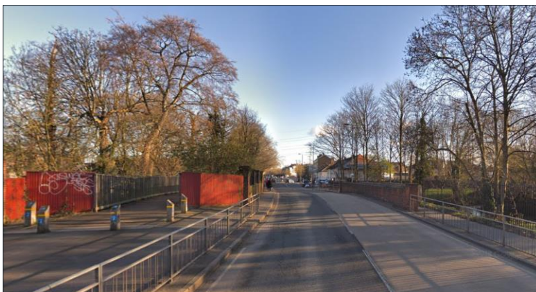
Figure 4 - View across structure towards north [Top - current view following collapse, Bttm – view prior to strengthening works]
