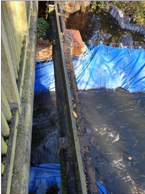
Figure 15 - Steel ducts containing BT Openreach services on East (Upstream) elevation
