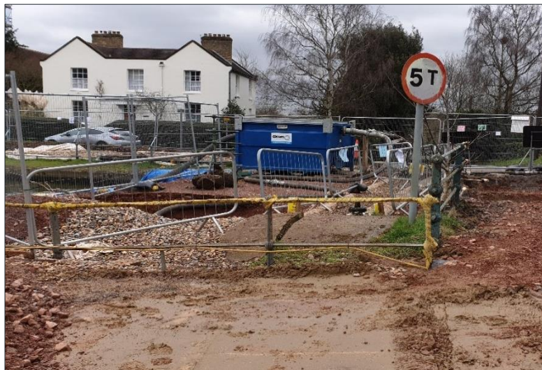
Figure 42 - Example over-pumping plant
