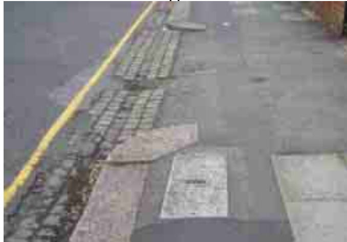
eg. covering of granite setts with tarmac, poorly patched pavement repairs
