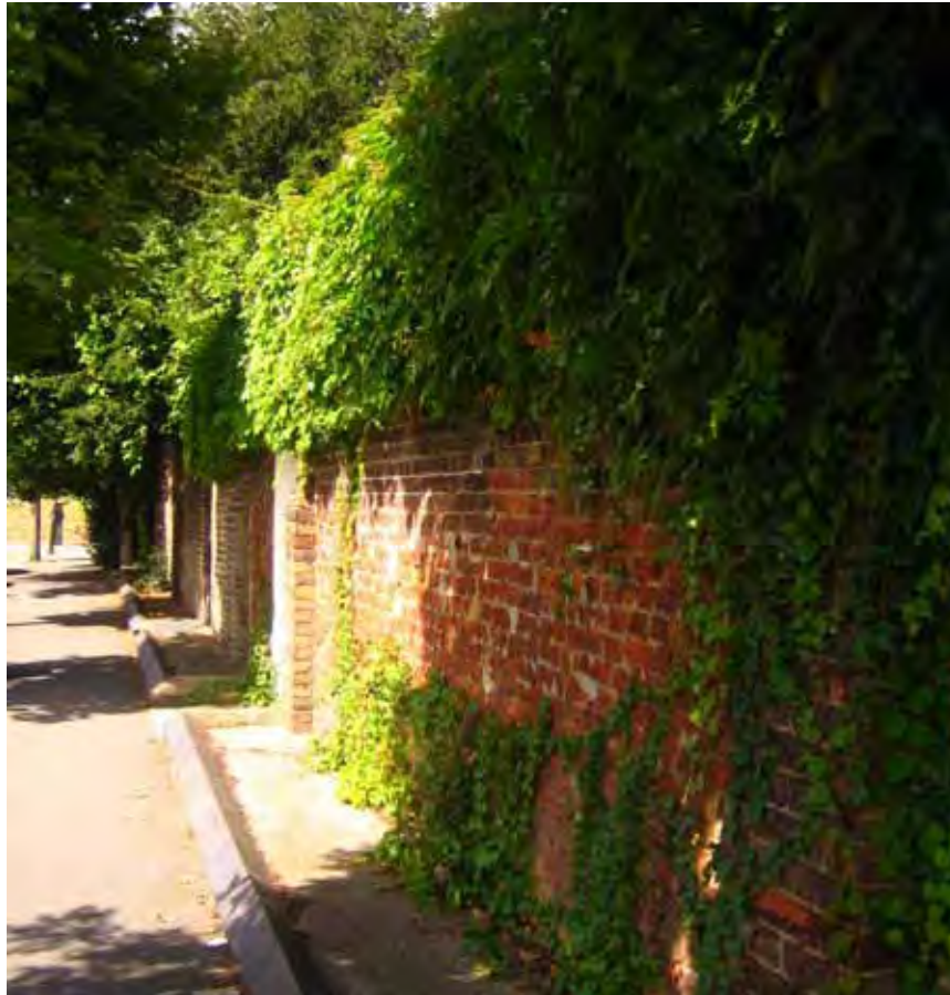
The high brick wall on the north east side has an unusual base design
