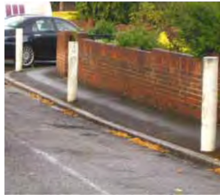
Poor appearance of metal bollards
