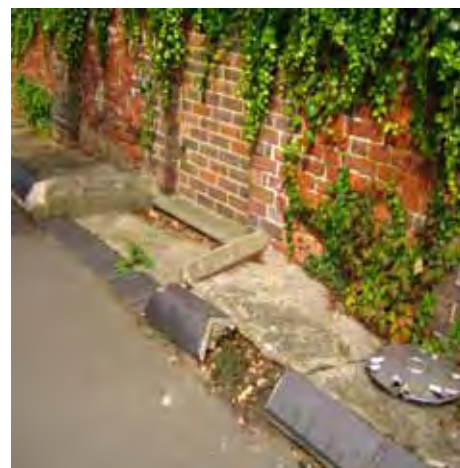
Poor condition and appearance of base of old wall
