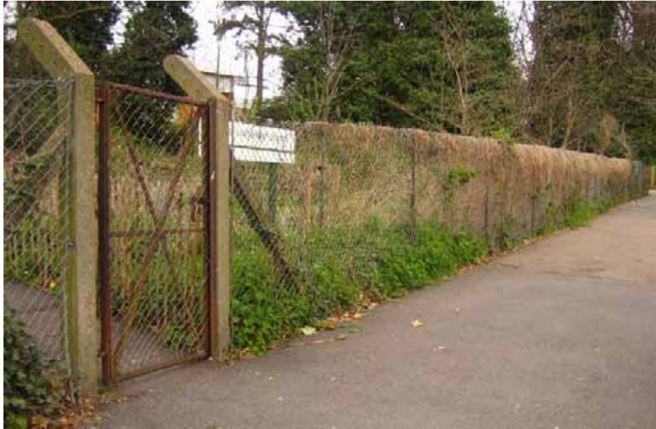
Poor boundary treatment to school grounds, Lake Road
