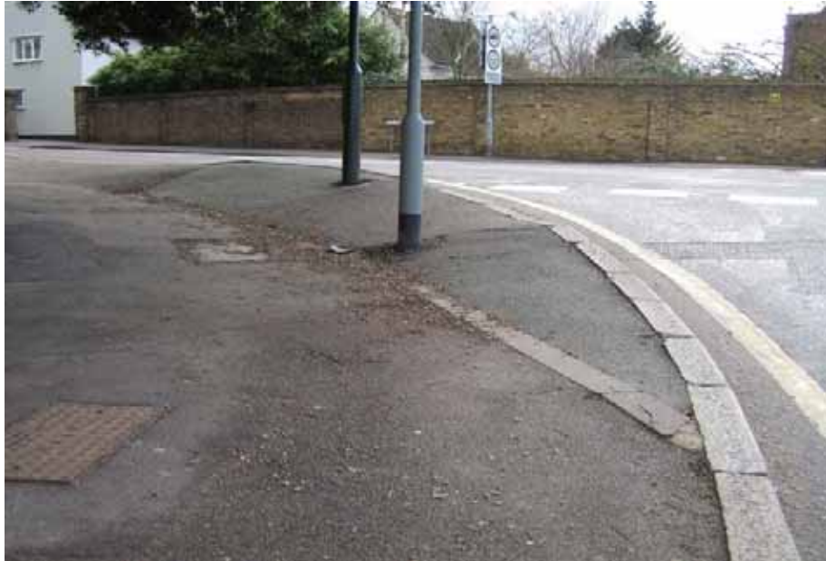
Poor pavement 'improvement'
