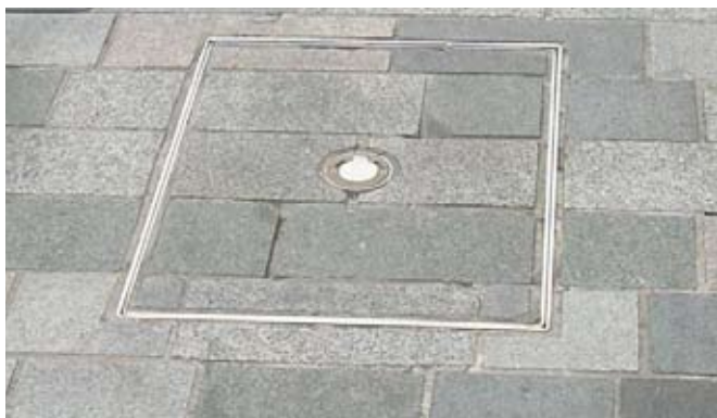
Recessed manhole cover lined-up with paving, and with neatly cut paving infill
