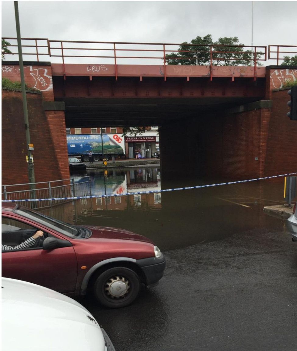
Figure 6.1: Extent of the flooding below Raynes Park railway bridge
