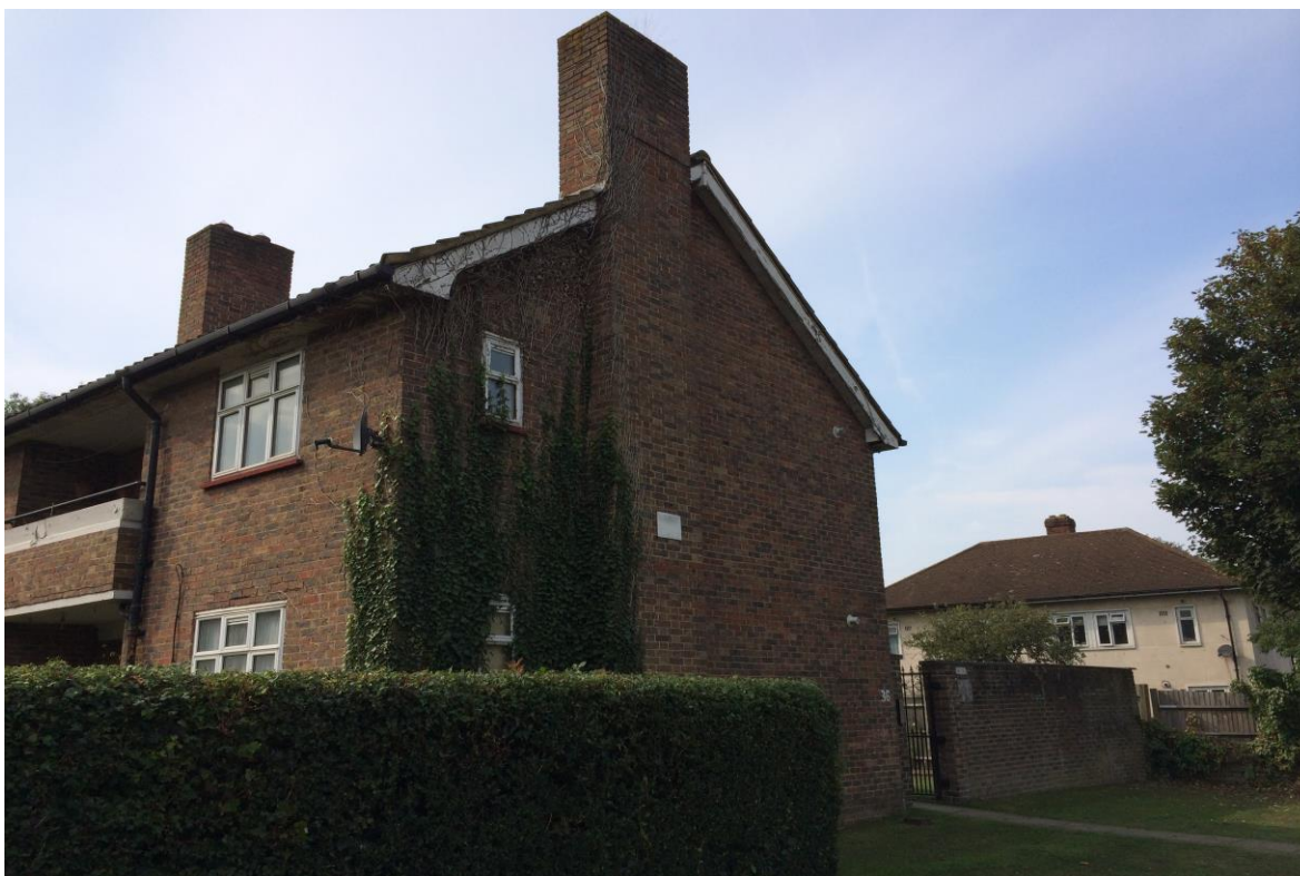
Photograph C12 – Vegetation to Side of Block 4 and Peeling of Paint to Eaves Board
