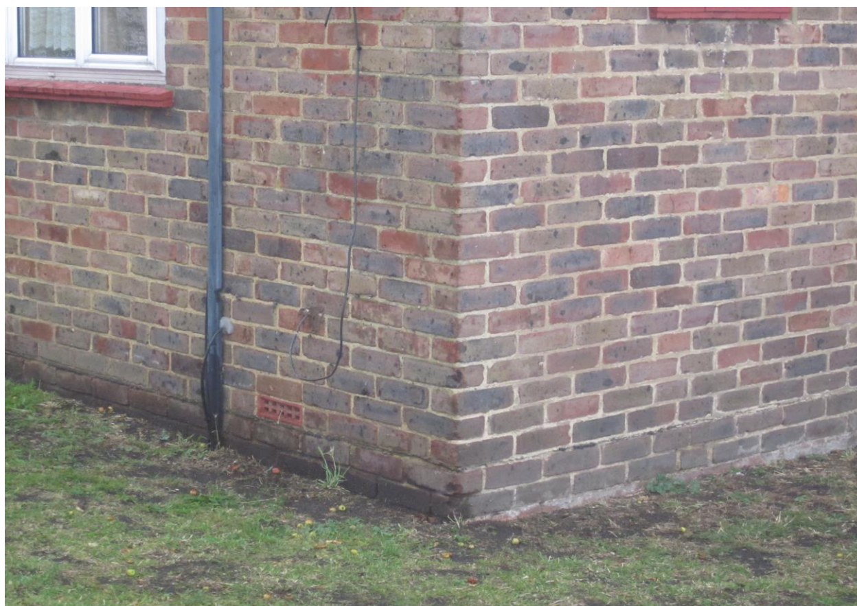
Photograph C2 –Ravensbury Grove Flat's Block- Air Brick at Ground Level
