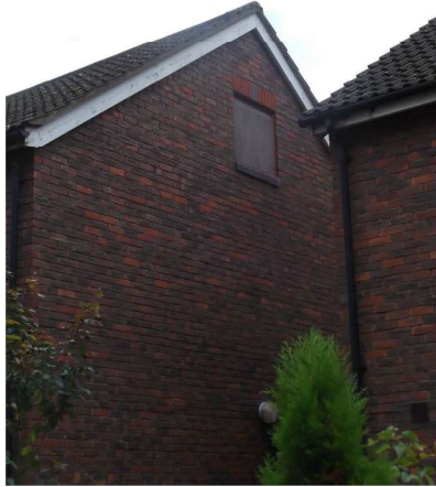
Photograph 5 – View of typical gable. Access hatches to roof voids are in poor condition and in need of replacement
