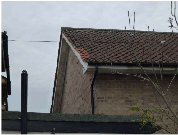
Photograph 5 – view of gable - Painted barge boards, soffit boards and fascia's all in need of repair
