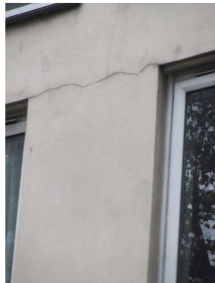
Photograph 4 – typical view of cracking in render
