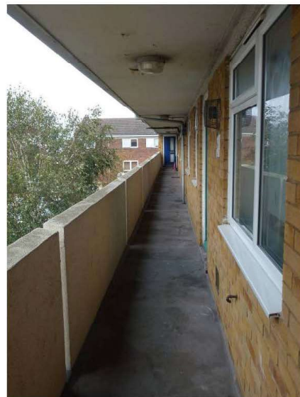
Photograph 7 – Tanner House - showing balcony access and concrete upstand balustrade with asphalt weathering
