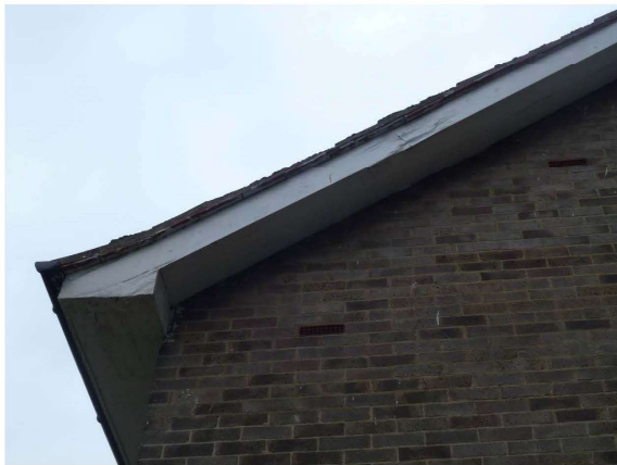
Photograph 6 - Rot in high level joinery.
