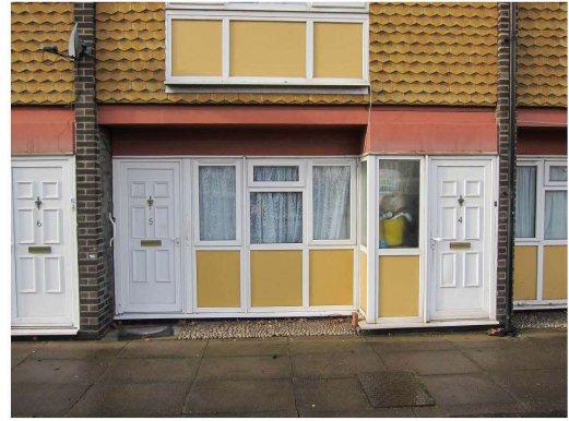
Photograph 2 – Entrance doors to ground floor flats and upper floor maisonettes. Exposed edge of first floor flats may form 'Cold bridge' detail.
