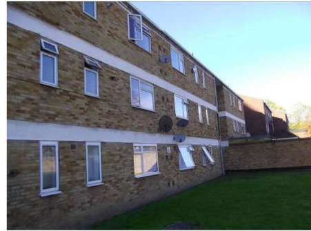
Photograph 1 – Mychell House - Rear elevation – Fair faced cavity brickwork and exposed floor edges
