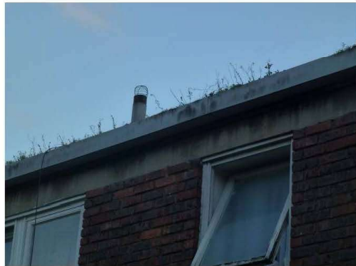
Photograph 13 – Eaves detail. Gutters need routine maintenance
