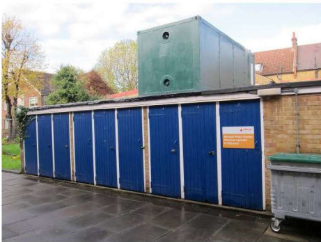
Photograph 12 – Hilborough Close Typical view external tenant stores – note roof covering in poor condition
