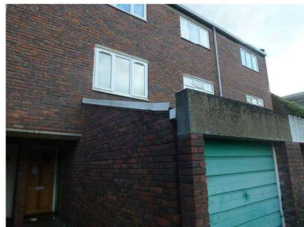
Photograph 2 – Typical view of garage projection, pitched roof and gutter behind the concrete parapet – note missing rainwater down pipe
