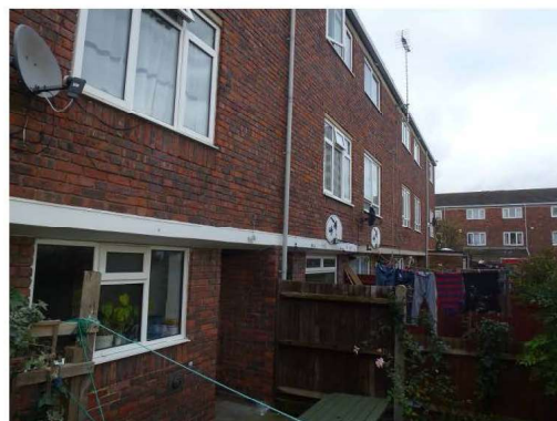
Photograph 4 – View of rear elevation and private gardens showing concrete slab at first floor level
