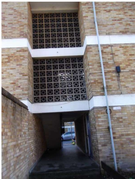
Photograph 2 – Mychell House – Communal entrance (No entry-call controlled doors and screens) block walling to stairwell areas.
