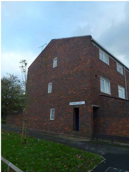
Photograph 7 – Gable end. Note missing sections of raised gable coping system and previous repairs
