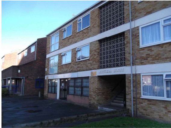
Photograph 1 – Mychell House - View of communal entrance to flats and ground floor office space
