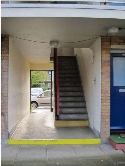
Photograph 9 – Hilborough Close Typical communal staircase. Note doors to entrance have been removed on front elevation. No doors fitted to rear.
