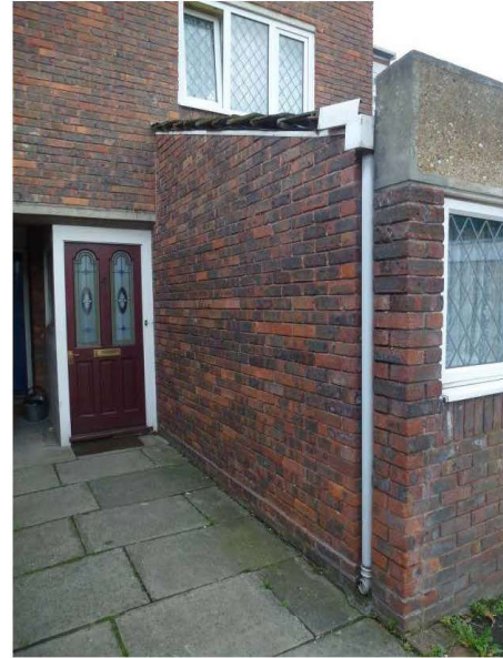
Photograph 6 – external view showing converted garage projection and sloping roof and gutter behind the concrete parapet with rainwater down pipe in place.
