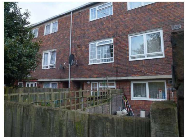
Photograph 9 – View of rear elevation and private gardens showing concrete slab at first floor level and timber garden fences
