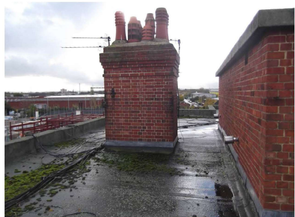
Photograph 15 – Typical view of chimney stack over Priory Close block. Some repairs to brickwork, pots and flaunching are required
