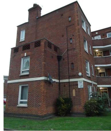
Photograph 2 – North end of Becket Close showing terraced roof area at second floor level.
