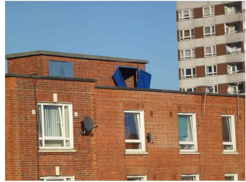
Photograph 14 – Roof top tank rooms on all three blocks. Doors have been left insecure and damaged by wind action. These should be rehung and made secure to avoid flying debris hazard and to avoid risk of frost damage to tanks and plumbing.
