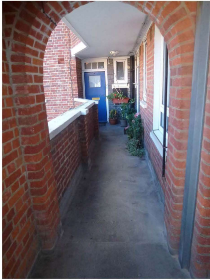
Photograph 13 – Typical upper level access balcony to flats showing asphalt weathering and brick balustrading
