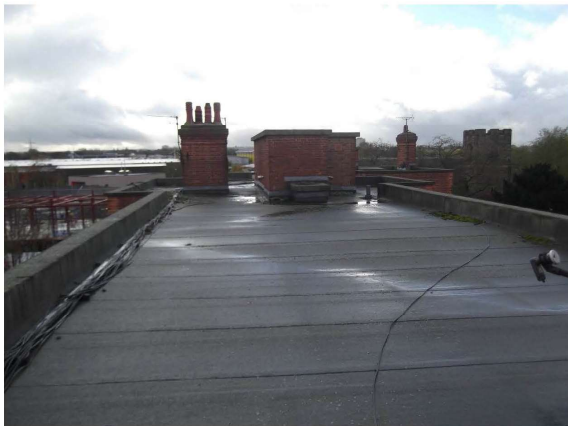
Photograph 14 – These blocks have been re roofed in the last 10 to 15 years with a High Performance felt roof system
