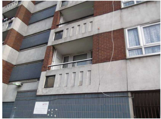
Photograph 6 – external view of private balconies and ceramic tile finish to ground floor and stairwell areas.
