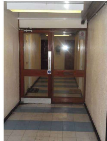
Photograph 4 – Typical internal common parts corridor. Fire doors are in need of overhaul and repair. Door closers need adjustment to close quietly and not require undue force to open doors.
