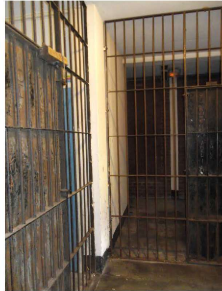
Photograph 24 – Security to tenants store areas. A review of the use of these areas may be required to establish if alternative use could be made of parts of these areas.
