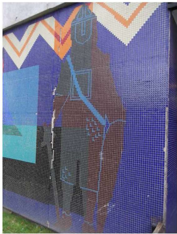
Photograph 3 – Each block has a decorative mosaic at ground floor level. These have areas of missing tile and are in need of repair.
