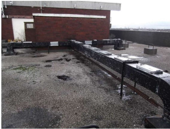
Photograph 9 – Roof over May Court. Asphalt is in fair condition for its age.
