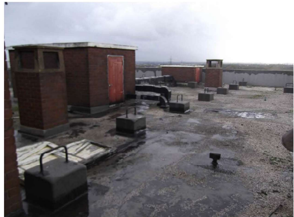
Photograph 8 – View of main roof over May House. This is likely to be the original roof covering applied when the roof was constructed in the 1950s and 60s. The levels of insulation provided in this roof will be low when compared to today's standards
