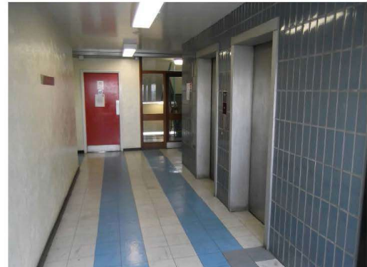
Photograph 12 – Typical upper floor lift lobby. Floor finishes on some levels have been damaged by flooding and are in need of replacement.
