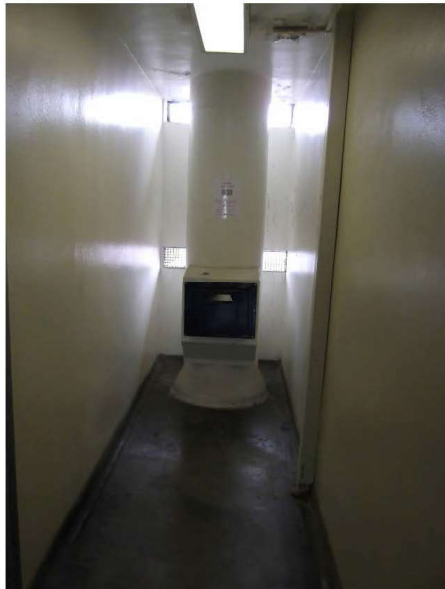
Photograph 15 – Typical view of refuse chute provided at each floor level. This arrangement does not allow for separation of recyclable materials at source
