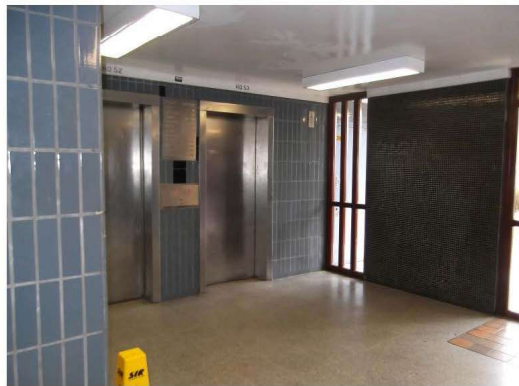
Photograph 11 – Typical view of entrance and lift lobby wall floor and ceiling finishes.
