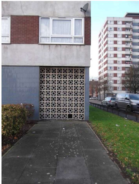
Photograph 7 – Typical view of concrete screen blockwork to ground floor tenant stores area.
