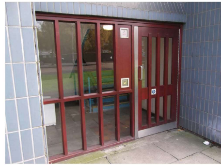
Photograph 10 – View of the ground floor fire escape from communal staircase. These screens would appear to be have been renewed within the last 10 years and are in good condition
