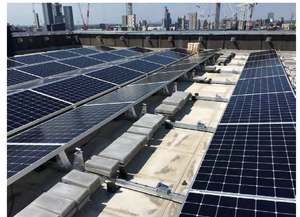
Figure 16 - Roof-mounted PV installations will have to be maximised. The panels selected should be high output and the concertina arrangement makes the most of the roof space available
