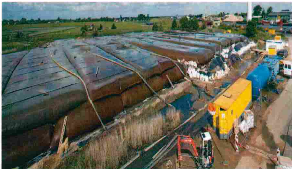
Silt bags being used to store silts until the material has dried and become more stable.
