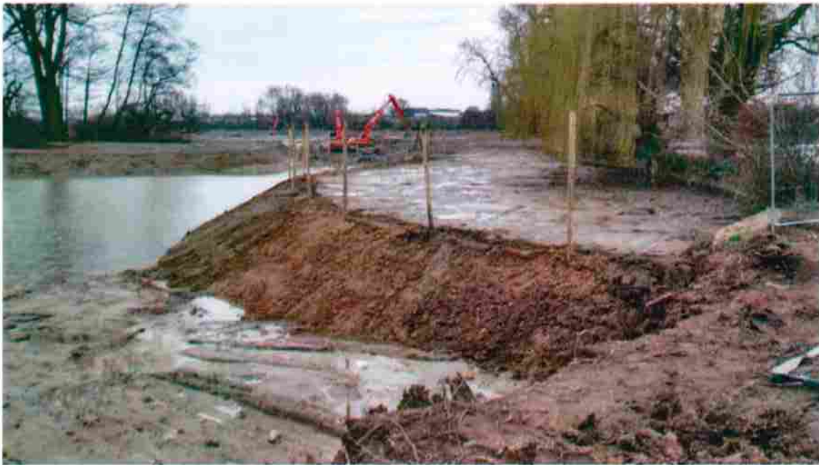
Excavation of the lake bed subsoils in order to create bunds, behind which dredged silts are stored.
