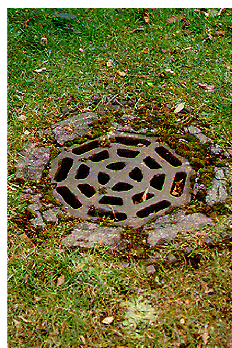
Cast Iron Drain Cover
